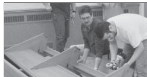
Moving & Installation tore down, helped load and then reinstalled all the finished pews at St. Theresa.
