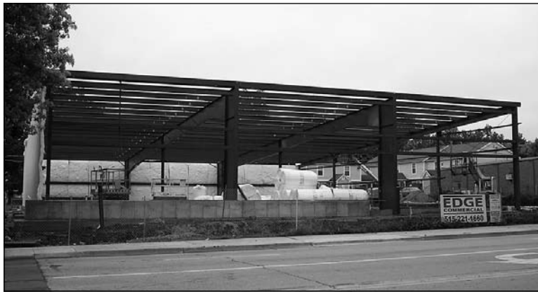
The new IPI Showroom is currently under construction at 1445 E Grand Ave. in Des Moines, just 2 blocks east of the Capitol Complex.
